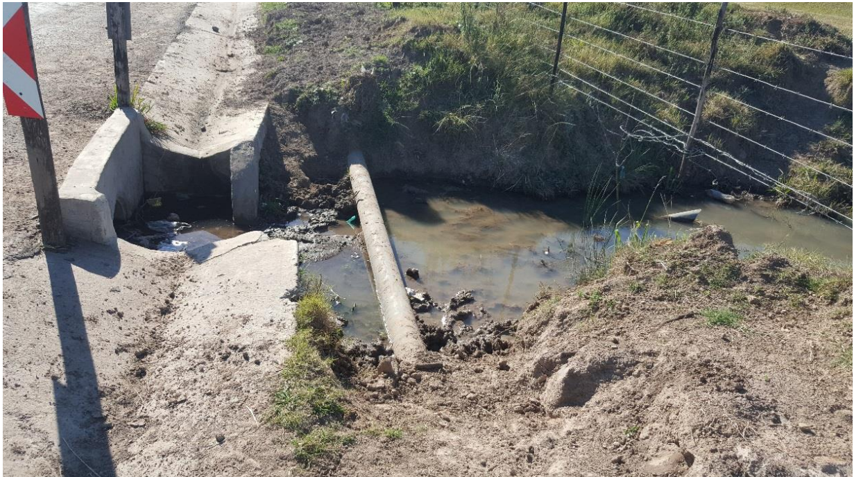
Figure 22: HDPE water pipe exposed to the ground
