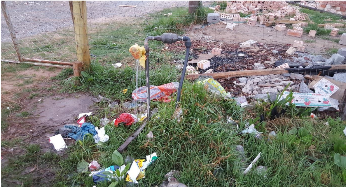
Figure 17: Leaking water meter strapped in with a plastic bag
