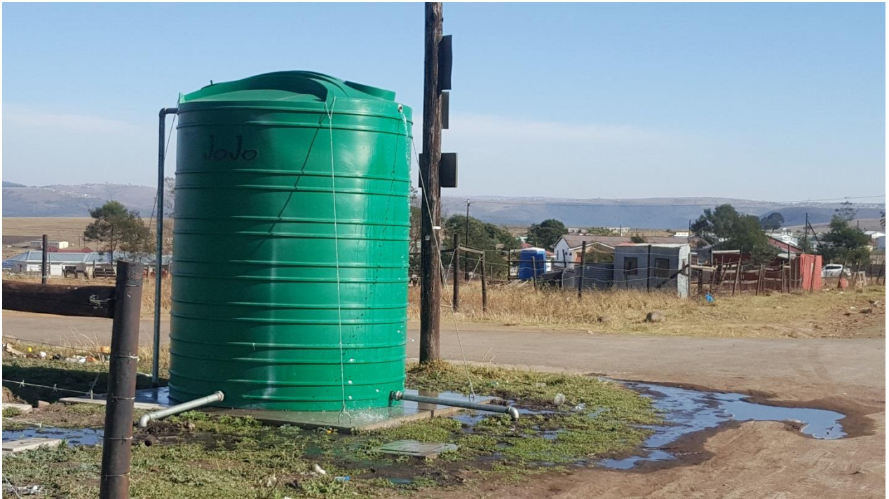
Figure 21: Unmonitored overflowing tank in Ibika
