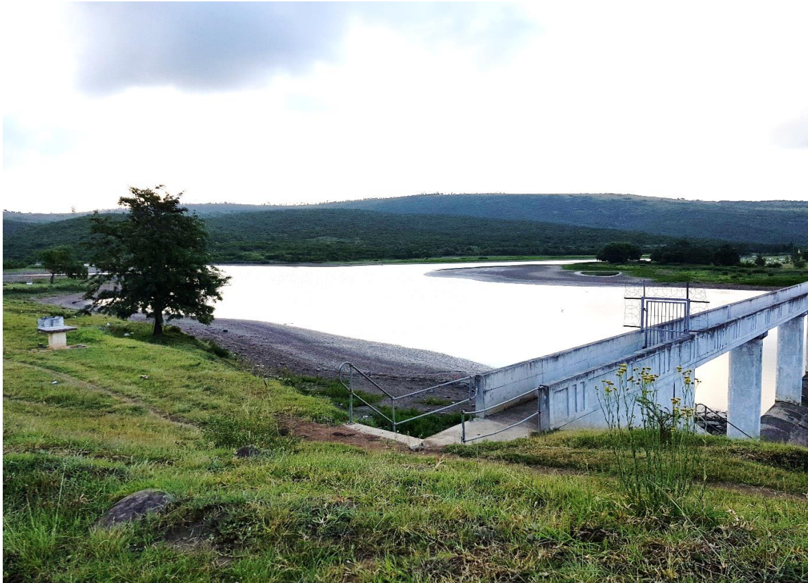
Figure 13: Silted Gcuwa dam in Butterworth
