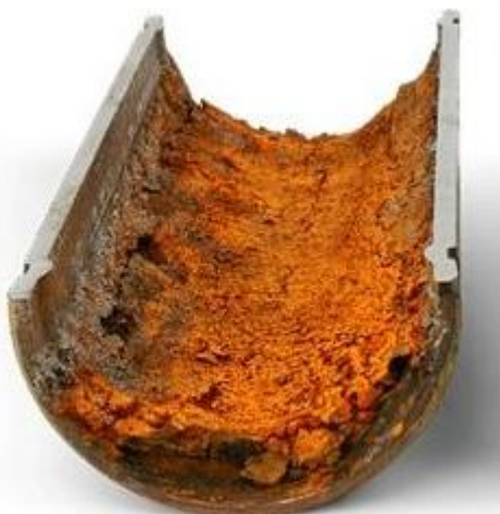
Figure 2.1: Pipeline Corrosion (World Iron & Steel Co., 2019)
