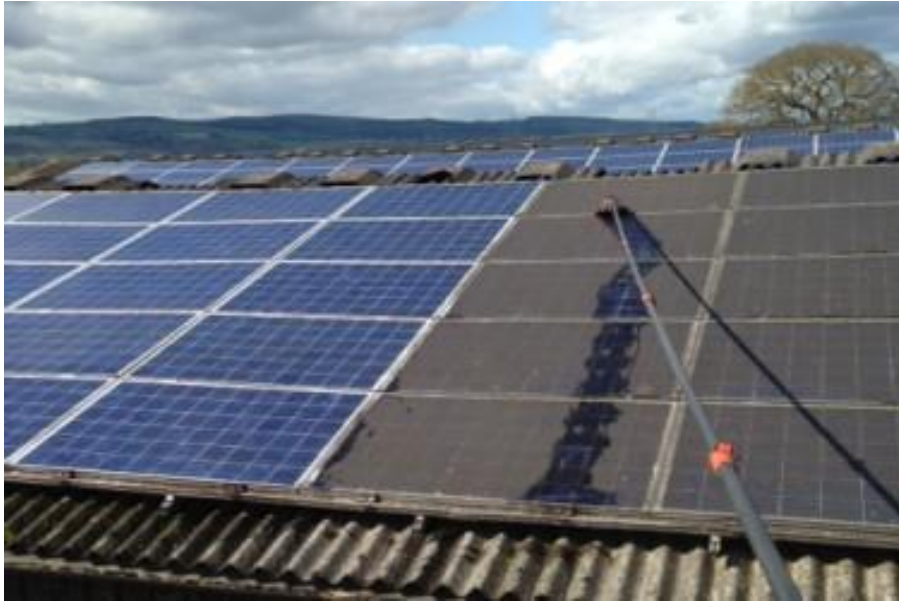
Figure 1.15: Picture of soiled solar panels in contrast to clean solar panels [45]
