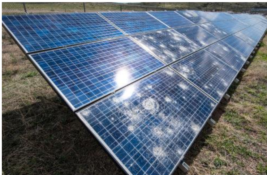
Figure 1.14: Picture of the damage to solar panels due to a hailstorm [44]
