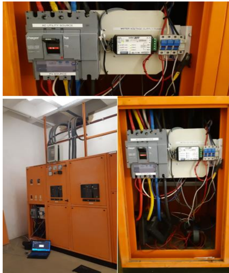
Figure 4.19 Set-up of the field data measurement at PCC
