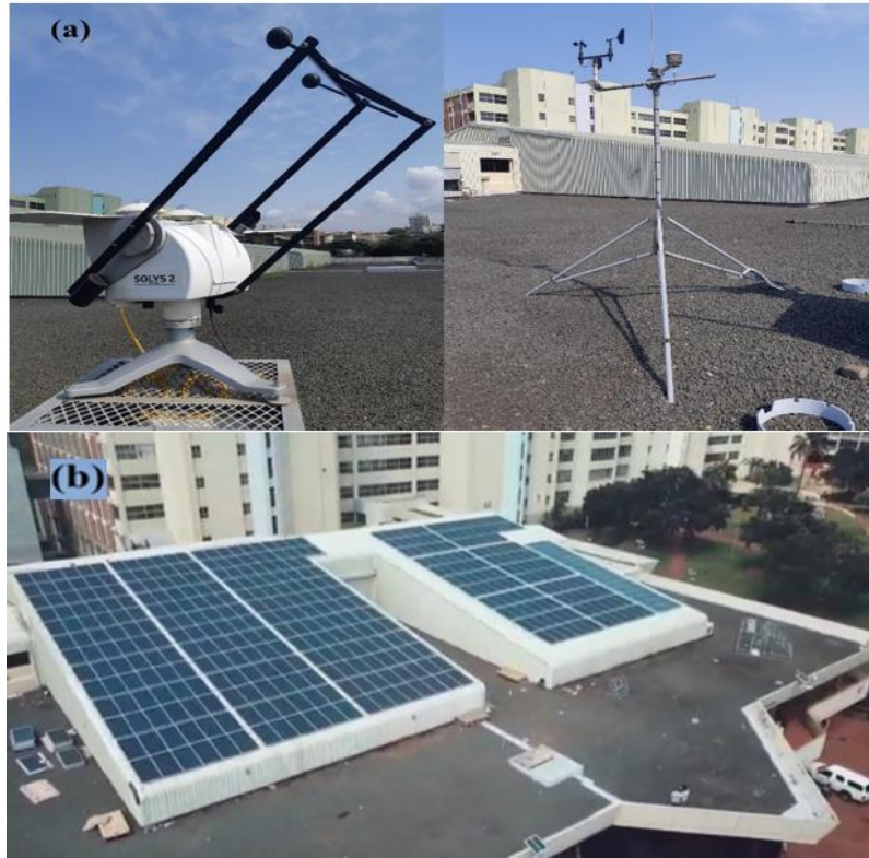
Figure 4.17 (a) Installed meteorological station (b) Installed PV array
