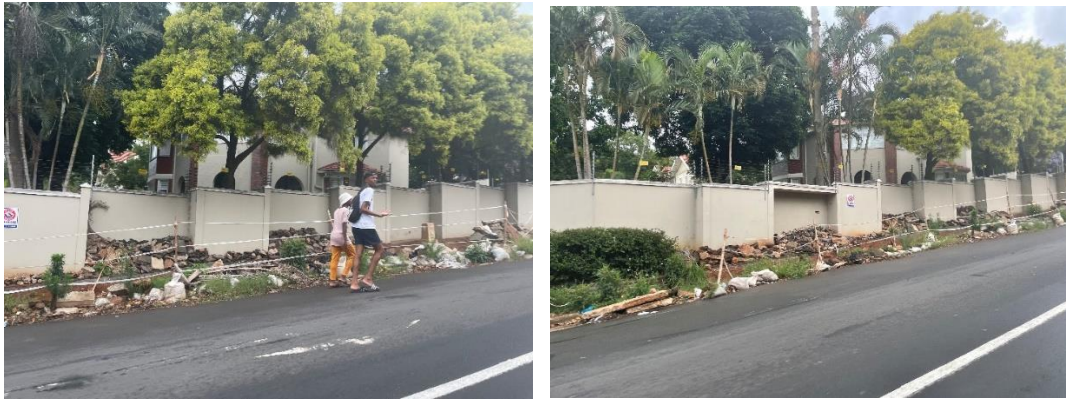
Image 1: Dug-up and unrestored municipal verge during fibre rollout at the corner of St Thomas and Peter Mokaba Roads in eThekweni (Source: Chetty 2022)
