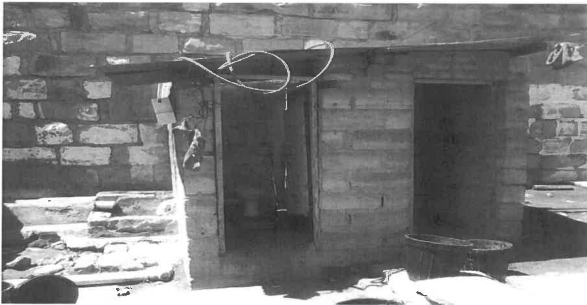
Picture 10: Pictorial view of conditions of the kitchen at MCCI
