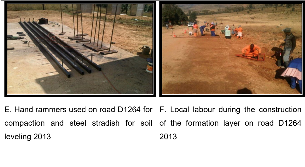
Figure 2. 8. A, B, C, D, E and F show tools and surveying techniques used during the LIC of the road D1264 formation layers
