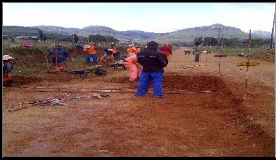
Figure 4. 1. Excavating to the top of the formation layer on road D1264 in 2013
