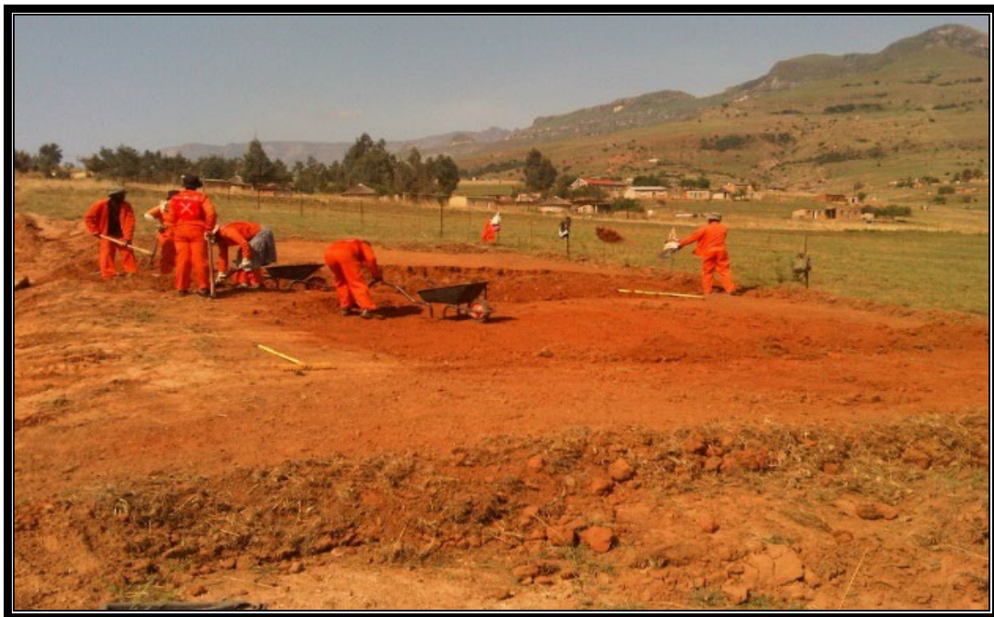
Figure 1. 2. Clearing and grabbing using LIC during the formation construction on Road D1264 in 2013
