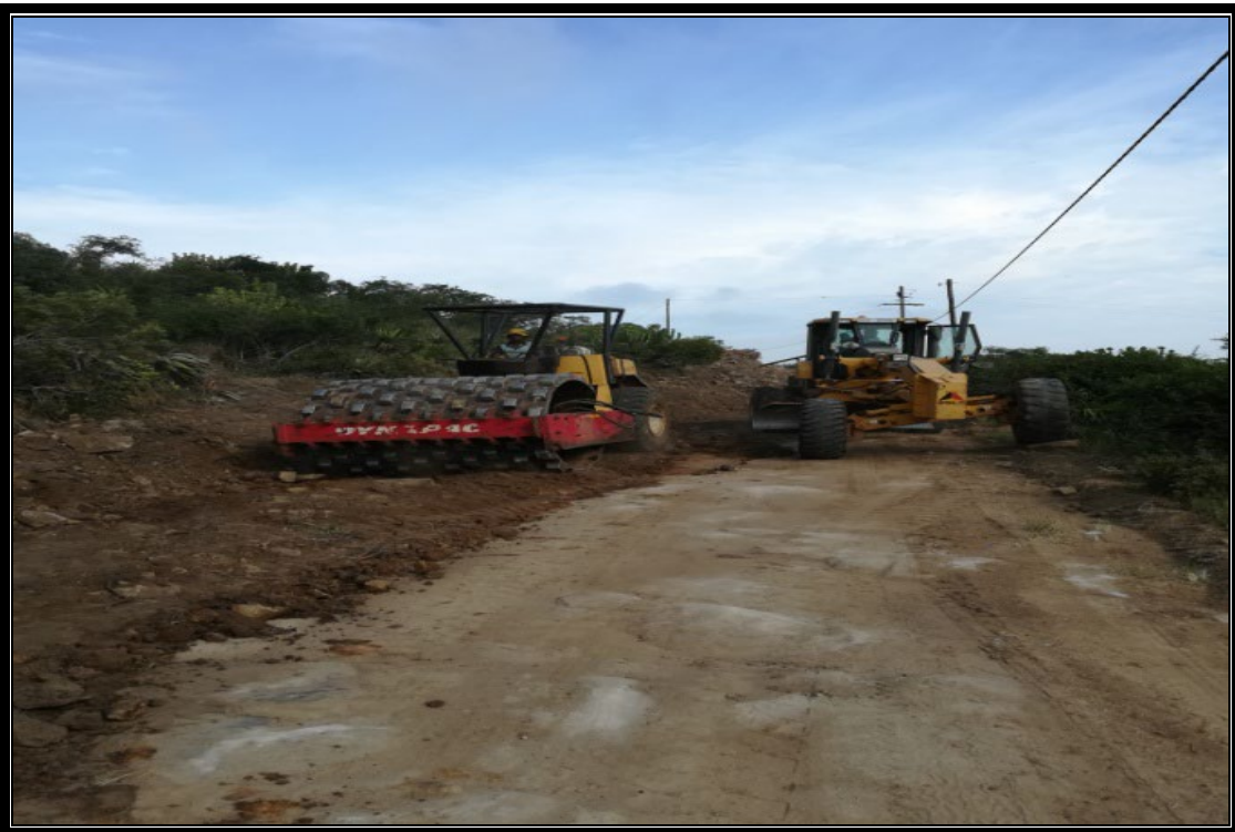
Figure 4. 4. Cutting levels and compaction with a grid roller and grader on road D1264 in 2013
