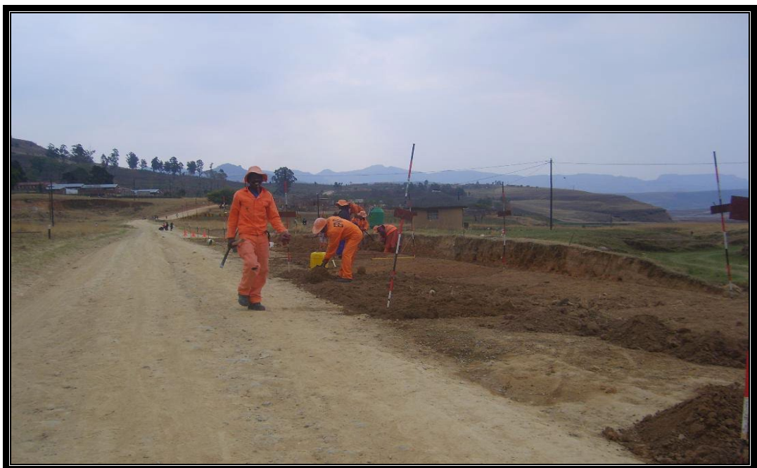
Figure 1. 4. Widening of the existing road using LIC during the formation construction on Road D1264 in 2013
