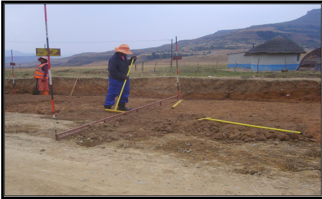
Figure 1. 3. Cutting of levels using LIC during the formation construction on Road D1264 in 2013
