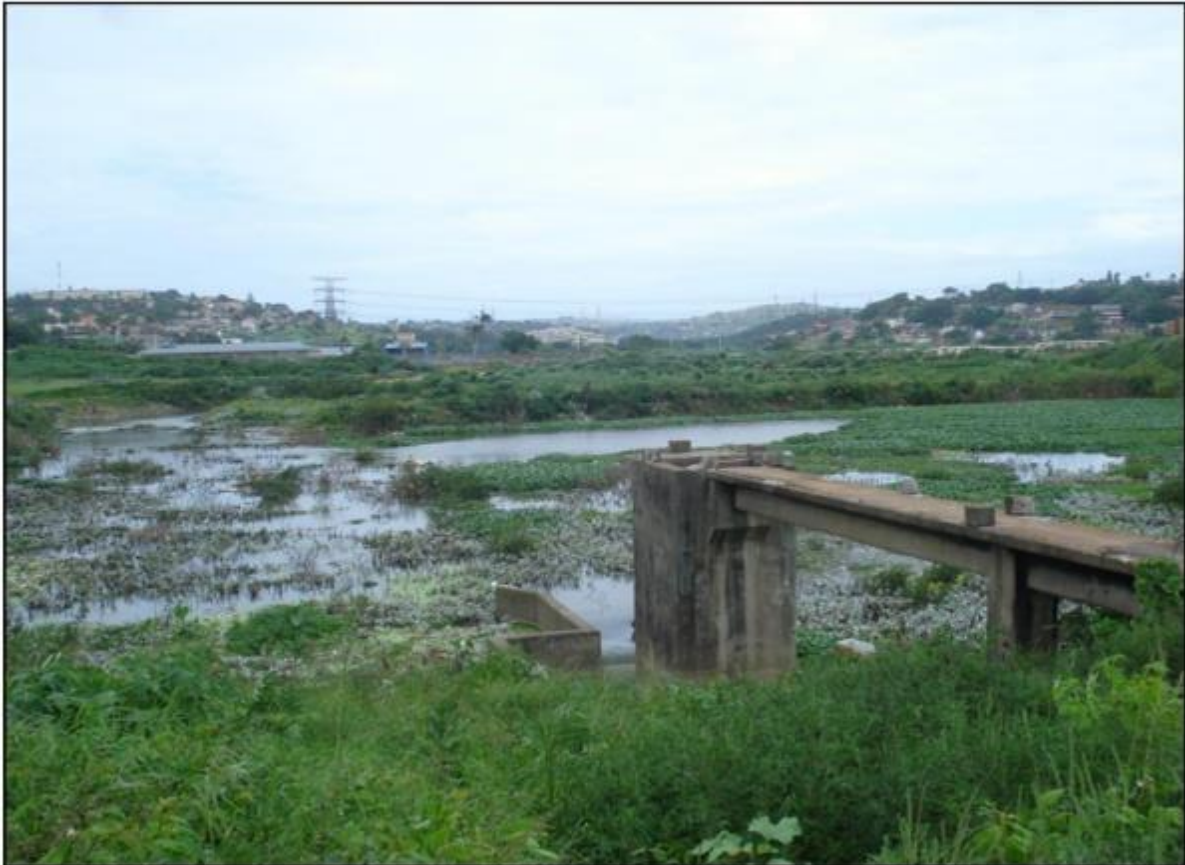
Figure 20: Sluice Gates at the head of the Prospecton Canal System.
