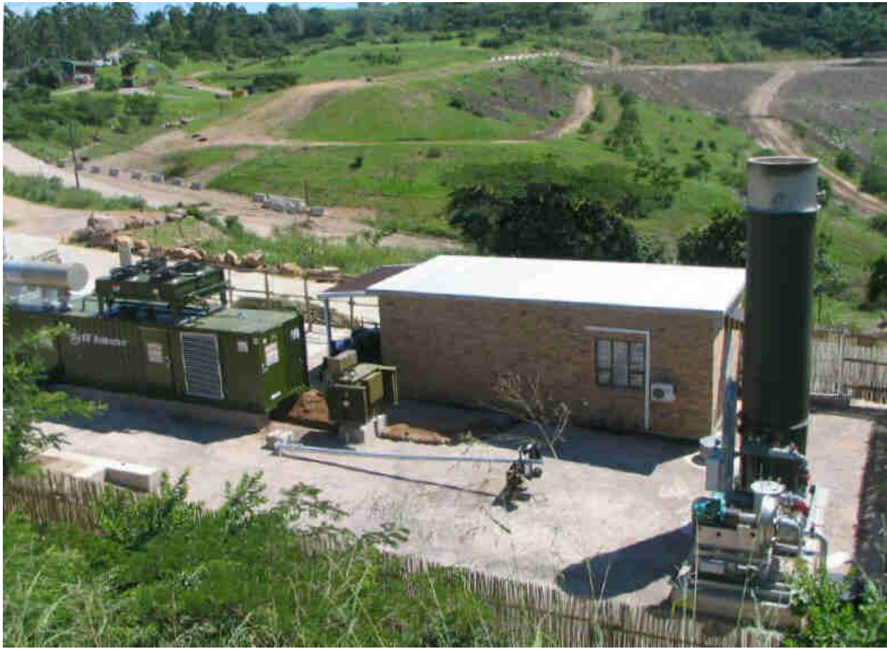
Figure 9: Marianhill Generator and Flare
