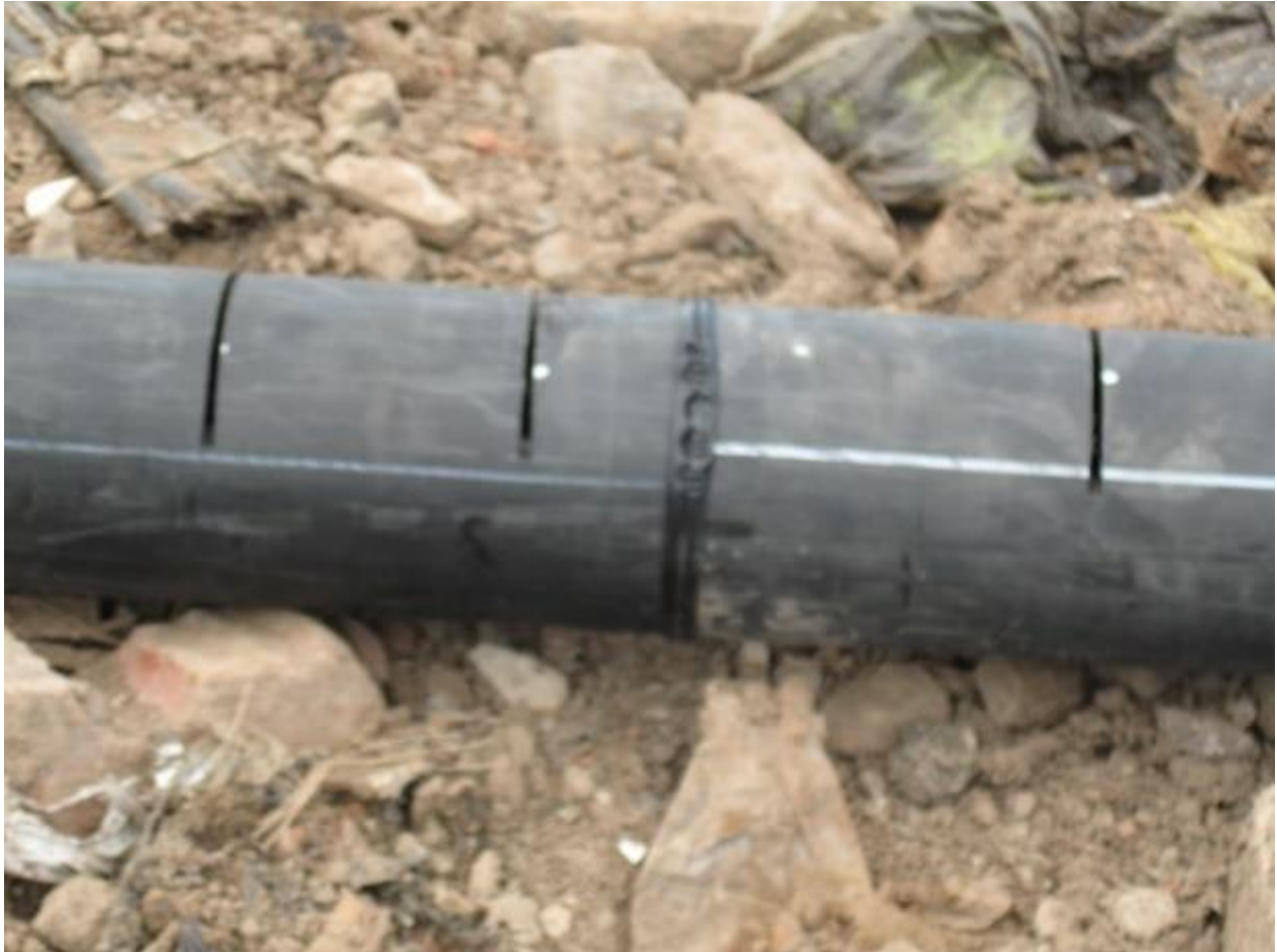
Figure 11: Sectional Incisions on Pipes Inserted Vertically or Horizontally into Landfills to Extract Bio-Gas
