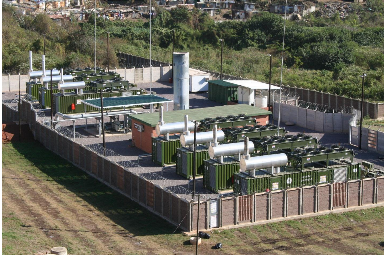
Figure 7: Bisasar Road Generators and Flare
