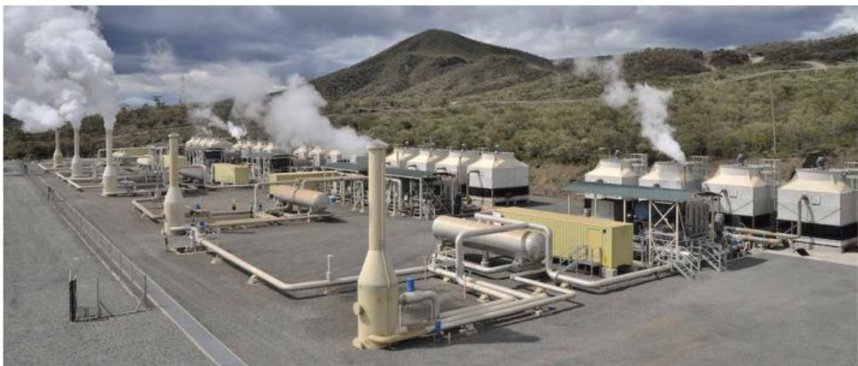
Figure 9-2: Photo of five Olkaria geothermal wellhead plants in Kenya[44, 58, 206, 347, 393, 394]
