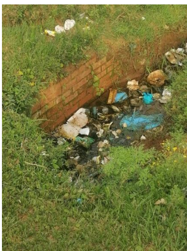
Plate 4: Waste trapped in a stormwater system in Mzinyathi (Photo: S Gwala)
