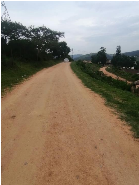
Plate 11: Gravel Road in Mzinyathi (Photo: S Gwala)
