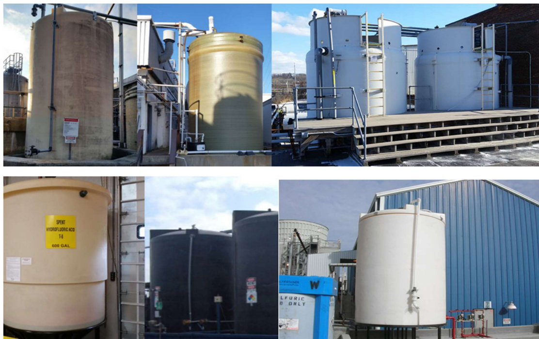
Figure 4: HDPE chemical storage tanks used in various chemical processing industries [36].
